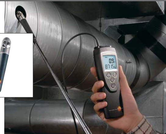
Monitoring air velocity in air conditioning ducts
