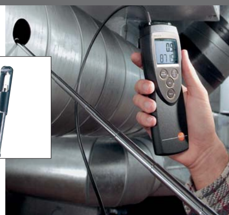
Monitoring air velocity in air conditioning ducts
