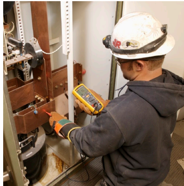
Checking incoming bus voltage and troubleshooting one of the mill’s primary breakers.
