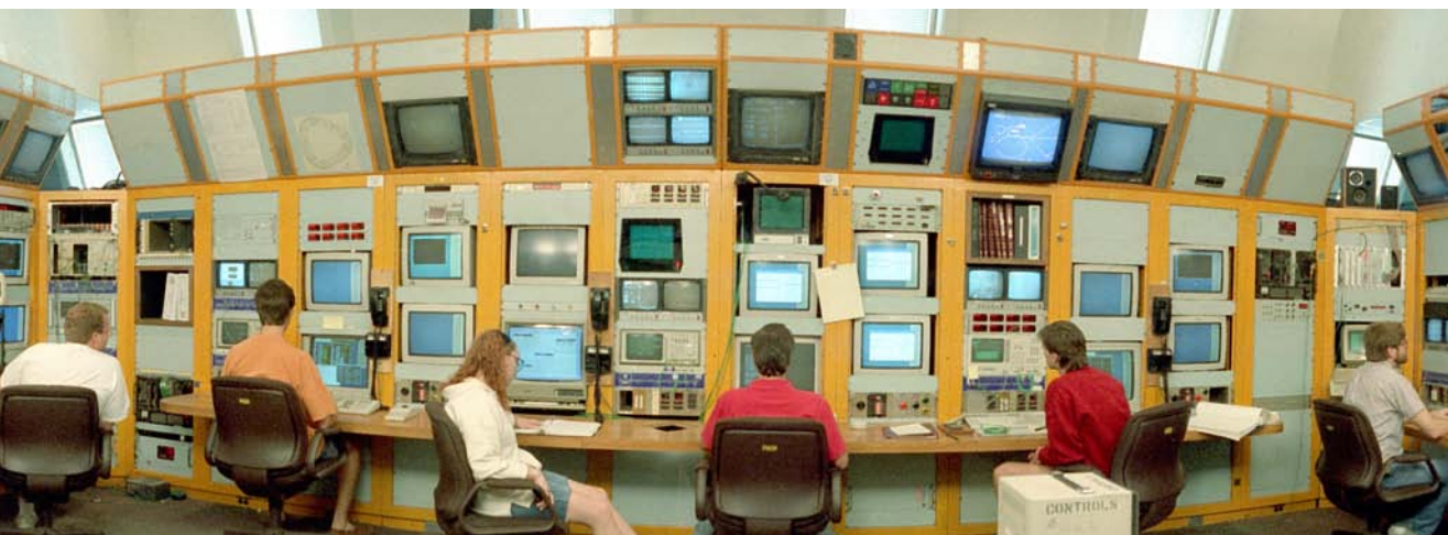
Main Control Room of Fermilab's Accelerator Complex
