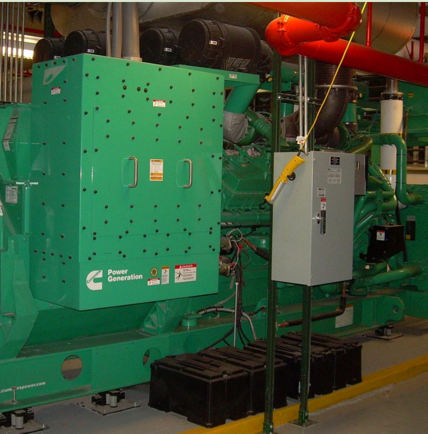
Large three-phase generators supply standby power to HVAC loads during loss of normal power. Such generators, quite often because of the large amounts of digital loads they must supply, may have difficulty maintaining sufficient power quality for proper VAV terminal operation.
